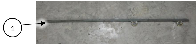
Figure 8 – Loose mount (1-MP-KW03.BP)
