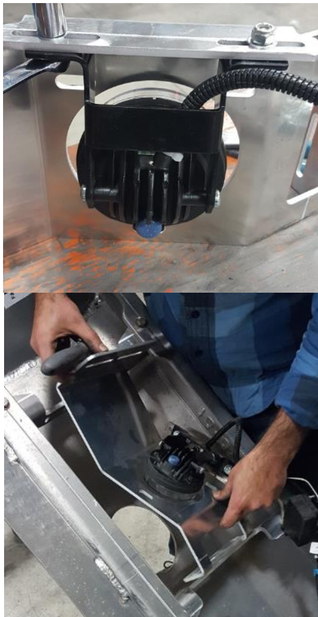
Figure 10 – OEM Light Installation (Passenger Side Shown)
